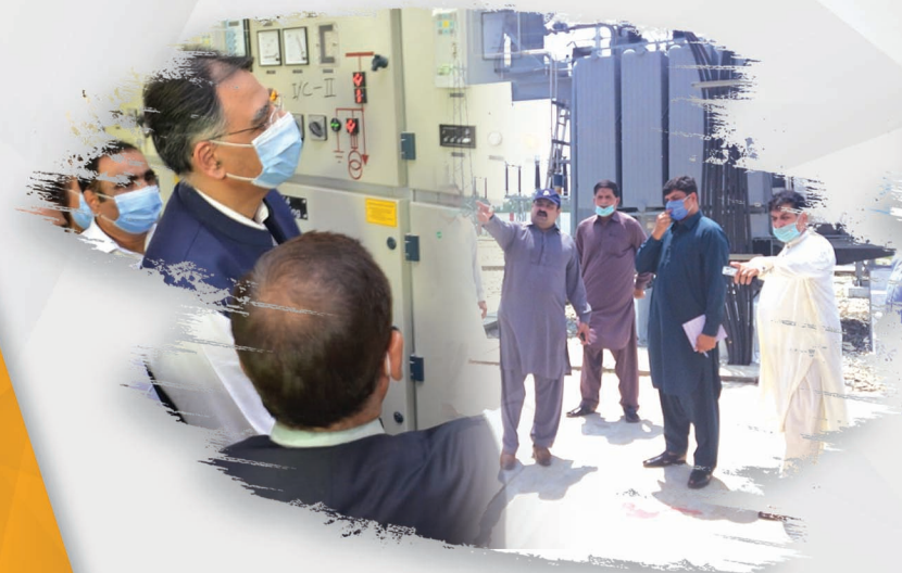
Grid Station Sector B-17 Scheme, Block - C
